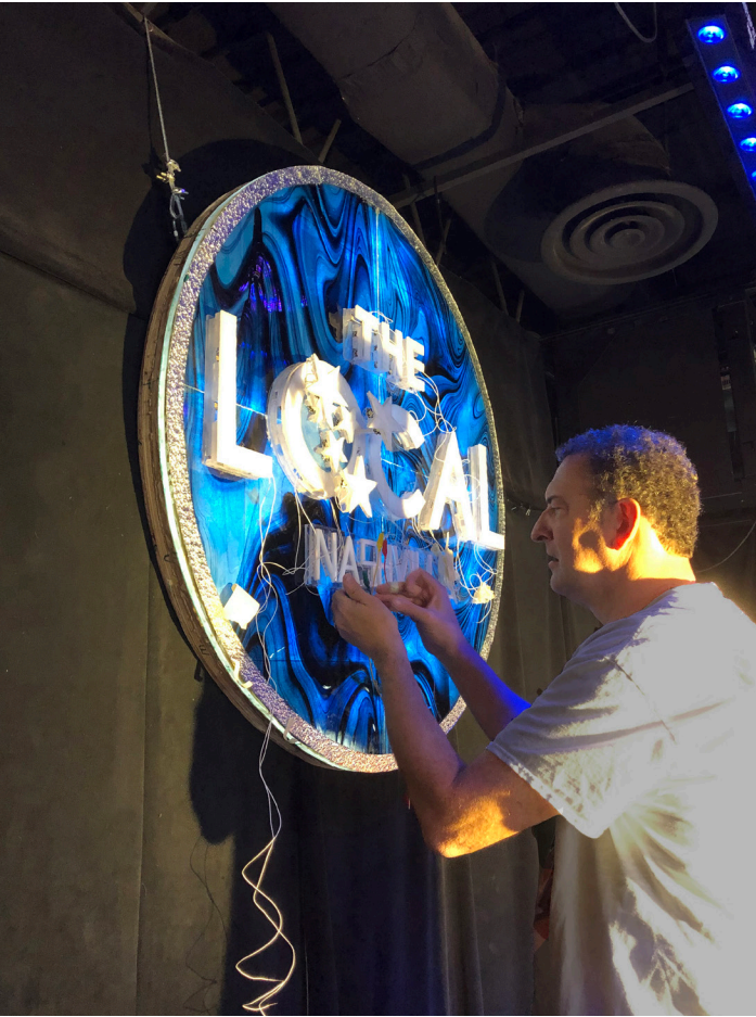
Paul Heller installs a stage sign at a Nashville live music venue, The Local.
